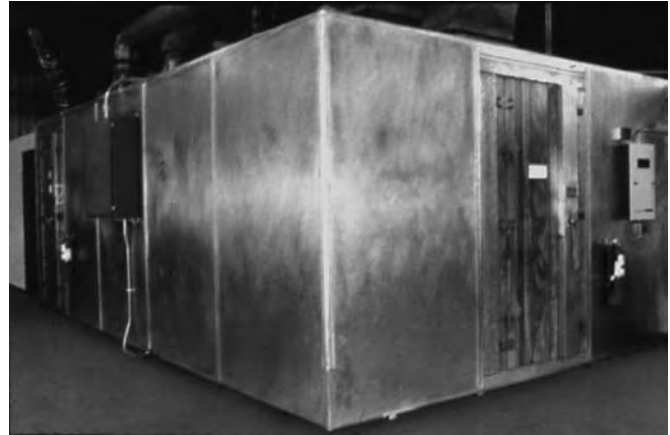
The Curtis screen room provides complete RFI isolation for equipment under test and the test instrumentation.
